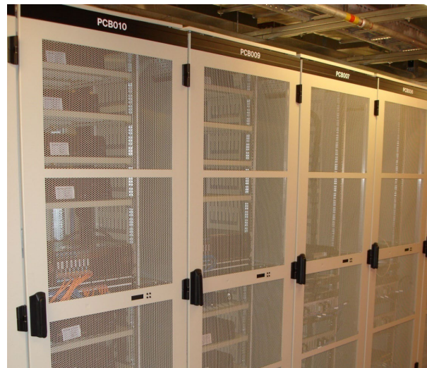
Figure 14-15 Cabinets Are Identified and Labeled
